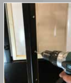
The wood frame can be used many times before it needs to be replaced.
